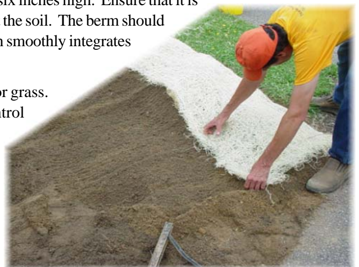
Erosion control matting made of coconut fiber is carefully placed along the berm to prevent erosion on the downhill side of the rain garden.
