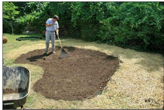
Fig 6. Leveling a rain garden to produce a flat bottom with sloped edges: a modified "bowl-shape" Photo by Bill Shuster, USEPA-RD
