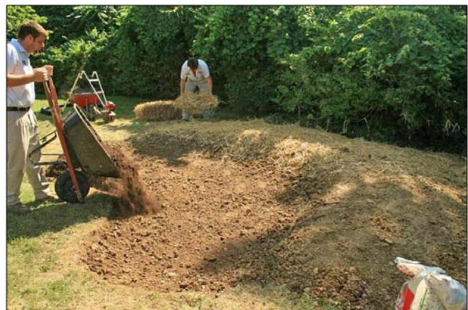
Fig 9. Adding soil and amendments to a rain garden Photo by Bill Shuster, USEPA-RD
