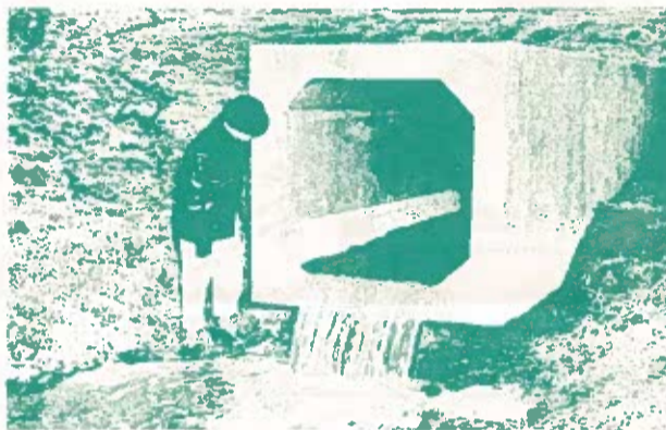
Temporary storage behind a dam plus regulated flow through the outlet prevents water "pile up" downstream.
