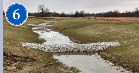
6 Swales (may include check dams) divert runoff.
