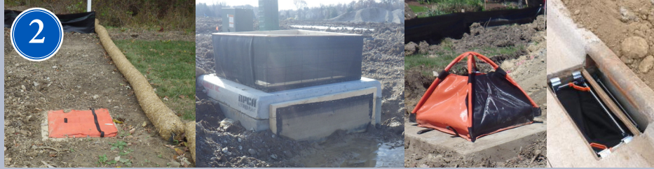
2 Inlet protection temporarily ponds water to filter sediment. Clean regularly and keep in place until site is stabilized.
